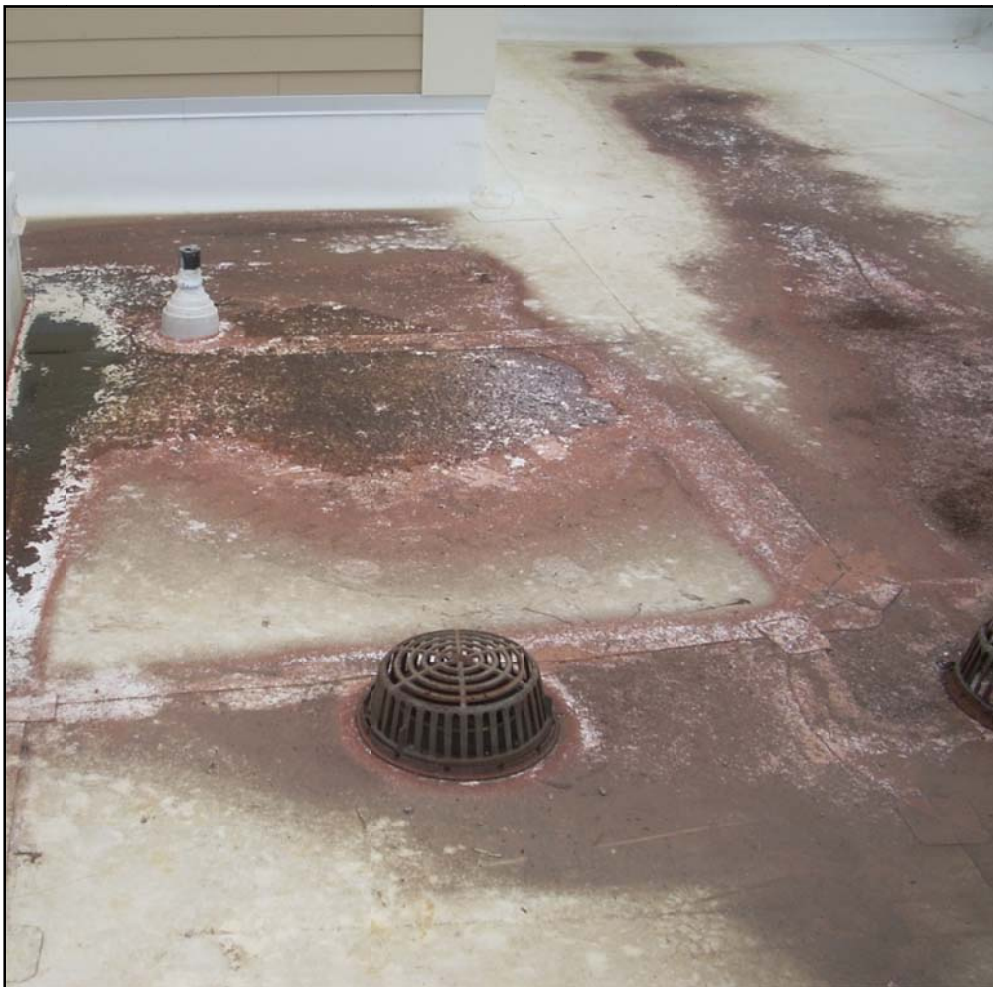
Red Algae growth on Thermoplastic membrane October 2013 Roof installed June 2013
